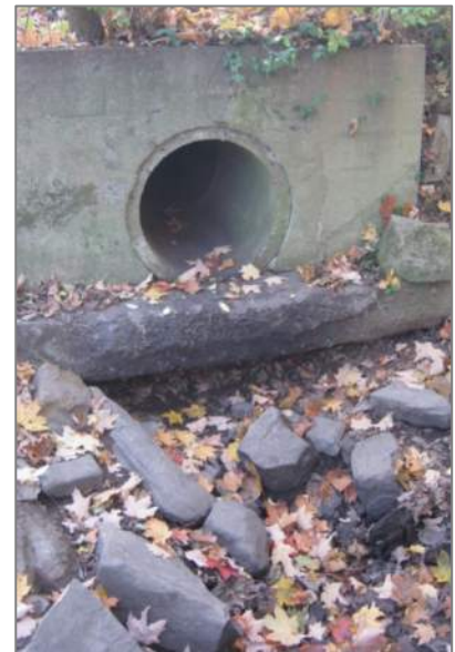
Photo : View of outfall #10 area during heavy rain events
